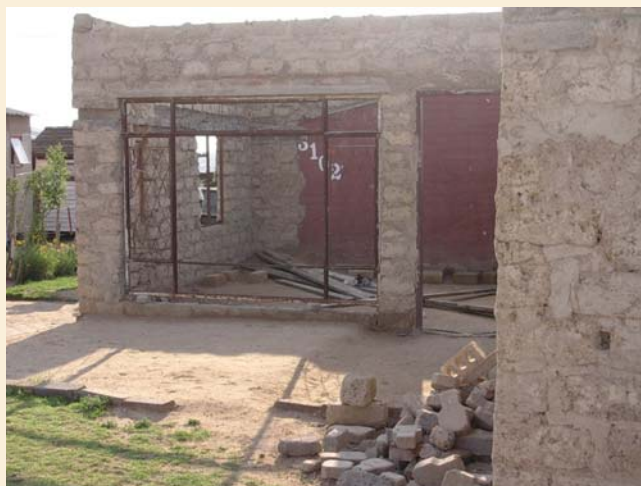
Building bit by bit to add a room on to an RDP house in Diepsloot, South Africa
